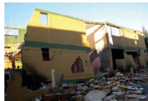
Image 2: A building with a collapsed ground floor as a result of the February 2010 earthquake in Chile. Source: Broze, Astoz and Yedlin, 2010 14 .
