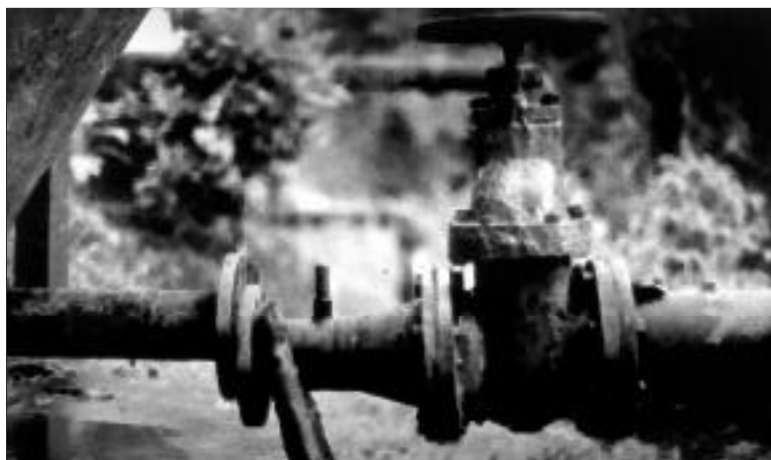
Certain damage can affect the quantity and quality of water supplied.
