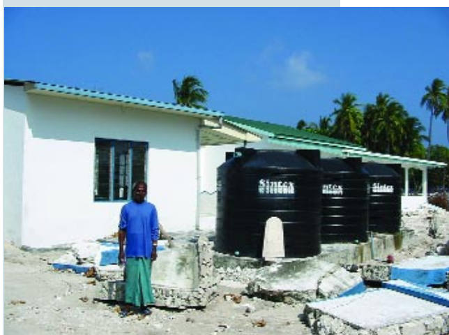
Water storage tanks in the Maldives.
