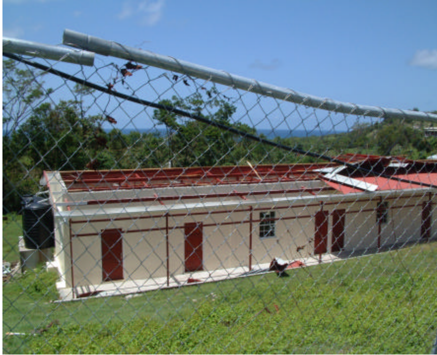
Figure 9 Damaged sustained by a school in Carriacou Photo Credit OECS Secretariat
