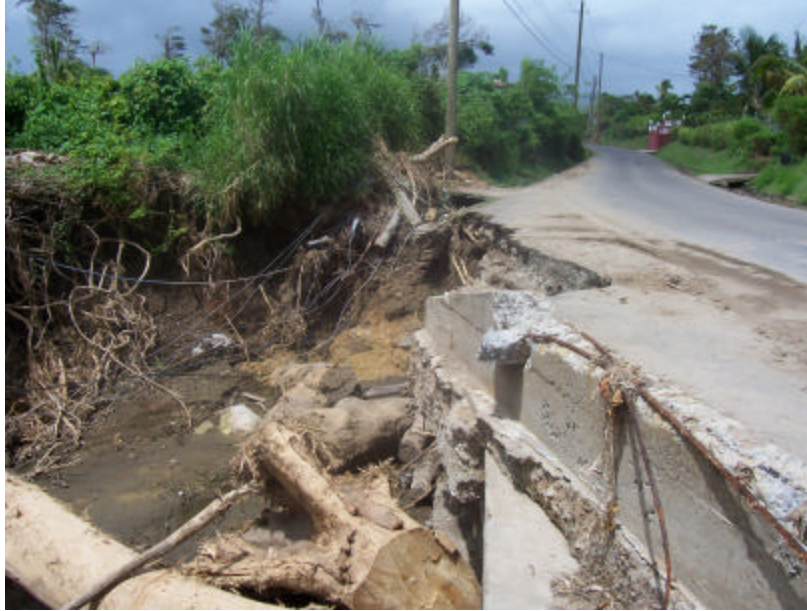
Figure 14 Damage to Approach and Structure of Pearls Seamoon Bridge Photo Credit Public Relations Officer, Ministry of Works, Grenada
