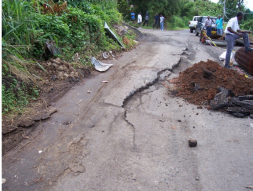
Figure 13 St. Paul's Land Slippage and Road Failure Photo Credit Public Relations Officer, Ministry of Works, Grenada
