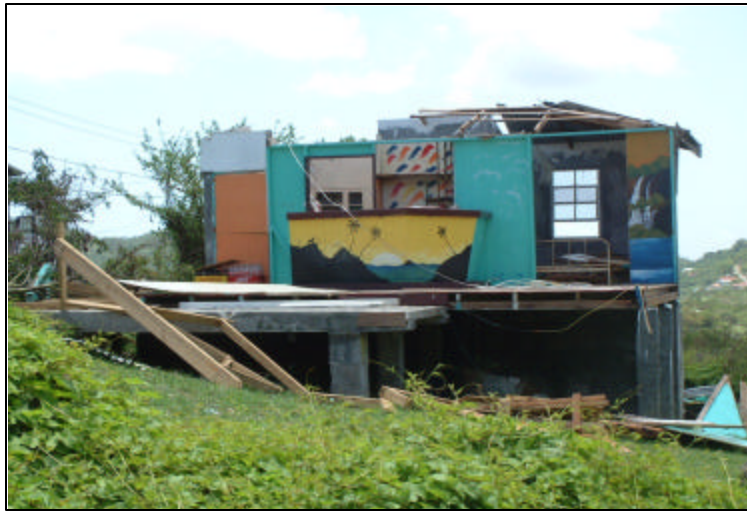
Figure 5. Damaged house in Carriacou Photo Credit OECS Secretariat
