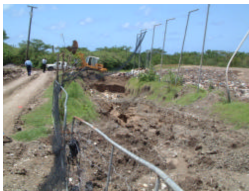
Figure 16 Erosion At Dumfries Landfill
