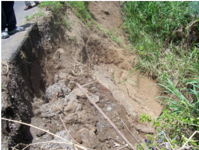
Figure 12 Debris obstructing Watercourse at Mt. Carmel Photo Credit Public Relations Officer, Ministry of Works, Grenada
