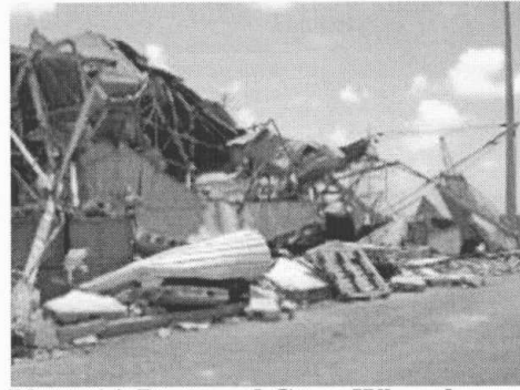
Photo 14 Damaged Geest Warehouse
