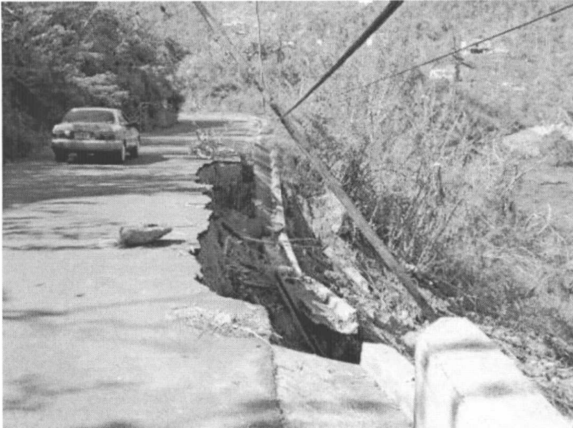
Photo 9 Erosion of Roadway at Westerhaul
