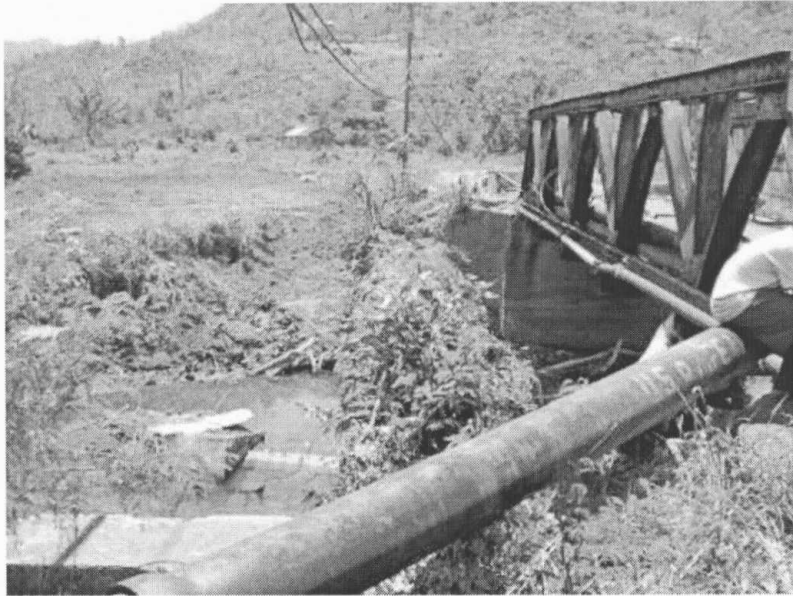
Photo 6 Damaged Water Supply Infrastructure at Beausejour
