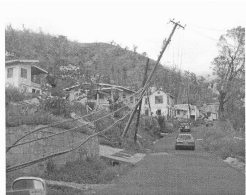
Photo 7 Downed Poles Carrying Communication Cables
