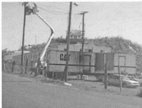
Photo 5 1.5 MW Unit in Lance Aux Epines
