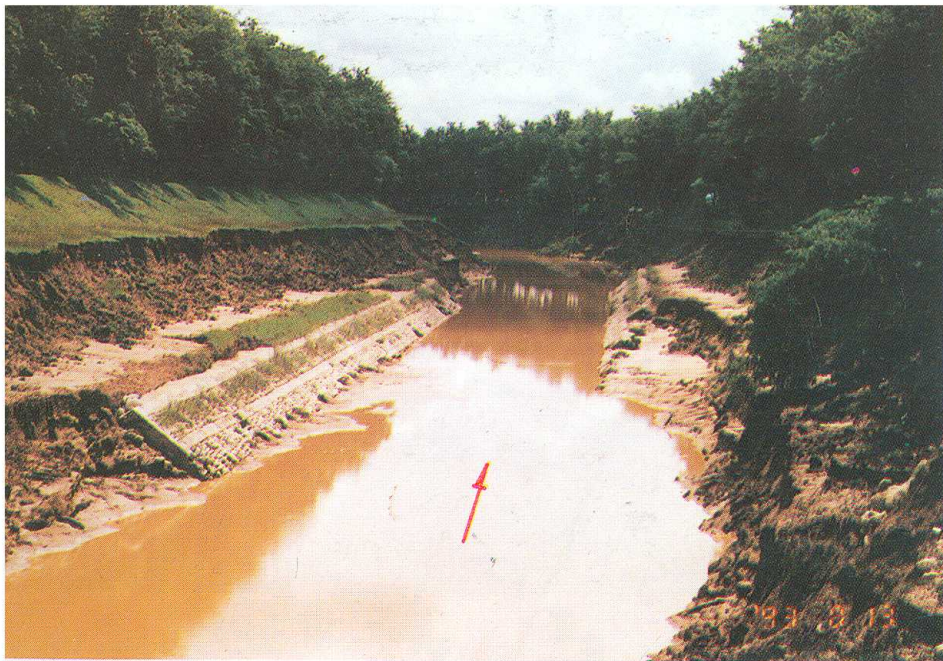
Erosion of East Main Canal.
