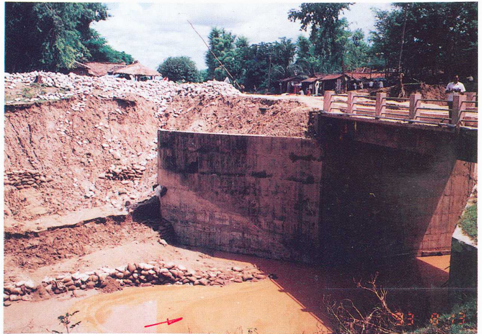
Damage to East Main Canal
