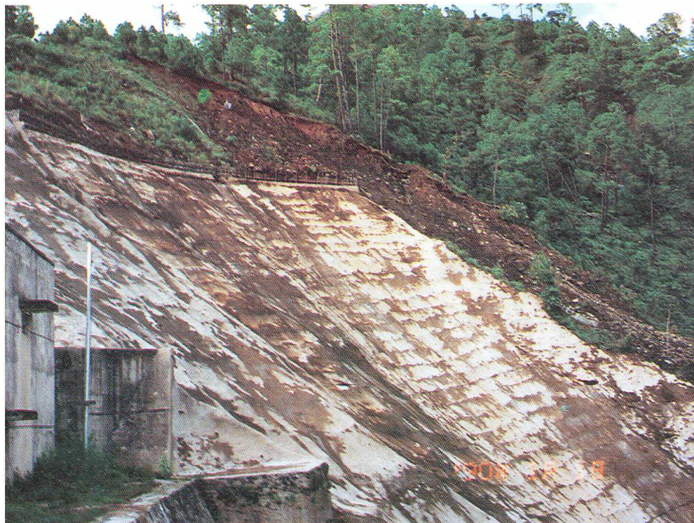
Slope protection works had been completed before the disaster and no damage was caused to the valve house.
