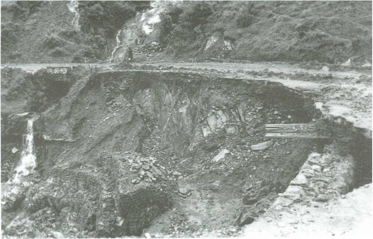
Landslide between Tistung and Palung
