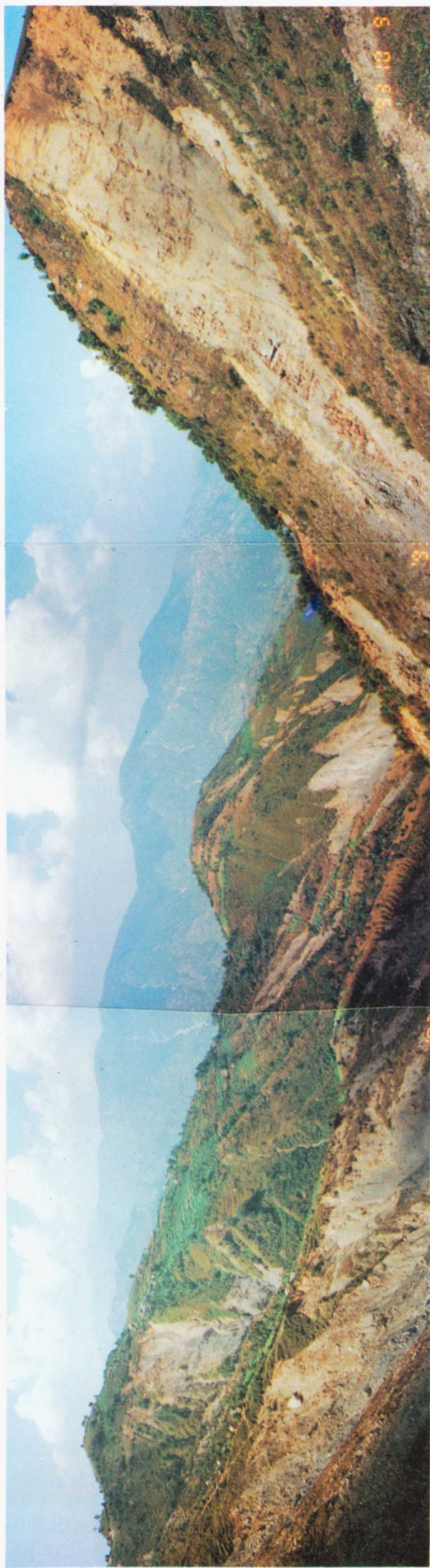
Upstream of Agra Khola at Chisapani where a major landslide is in active stage. Numerous slope failures are also seen in adjacent mountain range.
