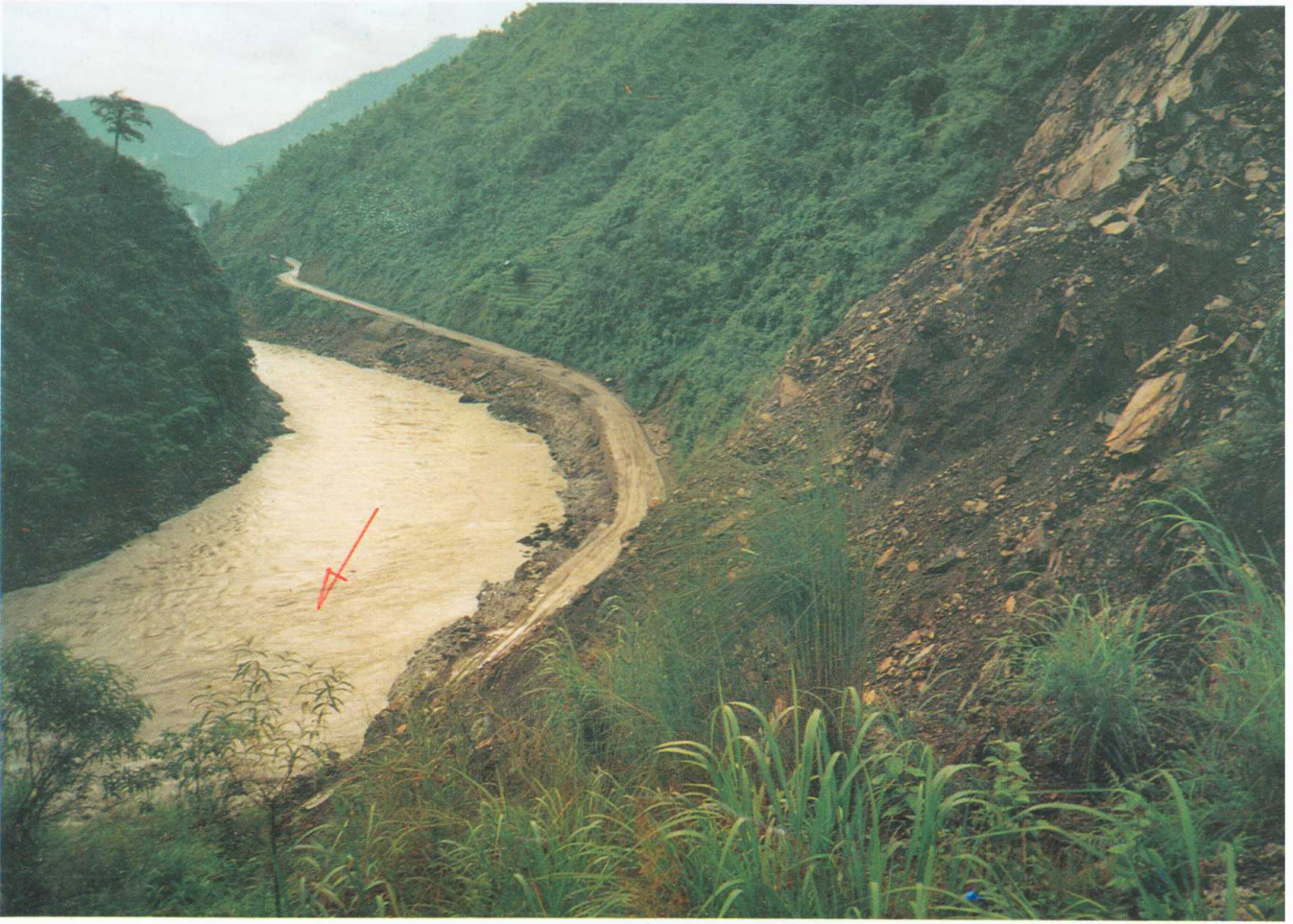
Jogimara Rockslide which blocked the road traffic for 3 days continuously.
