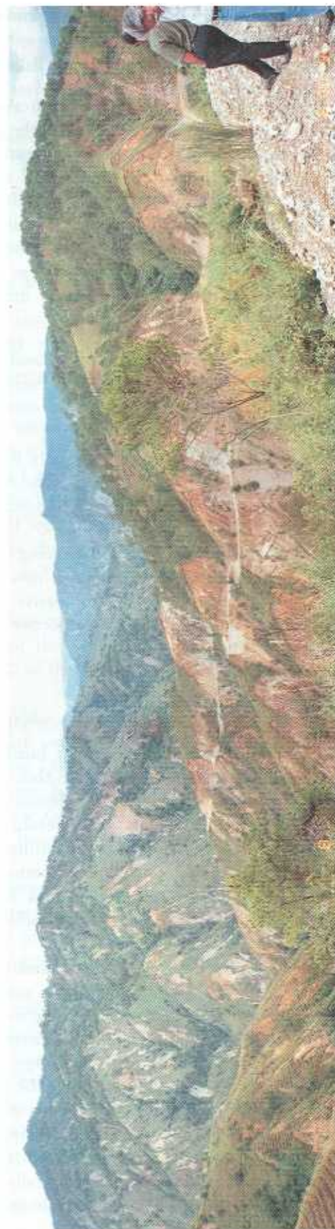
Fig. 6.2 Hilly landforms of the Caraballo Mountains with the typical shallow-seated landslides (debris slides) along the Dalton Pass Road (top). Shallow debris slides near the road leading to Ambuklao Dam (Cordillera Central), NE of Baguio (bottom).
