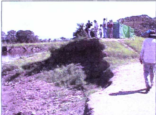
The levee along the Rio Chamelecon overtopped and breached in several locations.
