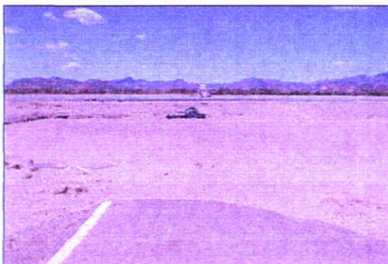
The entire left abutment of the bridge north of Choluteca was destroyed.
