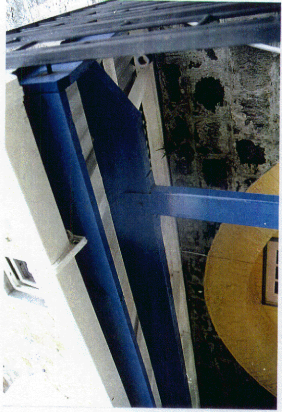
Photo 28: Inadequate details on shelter roof (previous photo). Steel column has actually been split at the topmost four corners. It is nailed to timber beam on the underside and bolted on the sides. Some bolts were missing.
