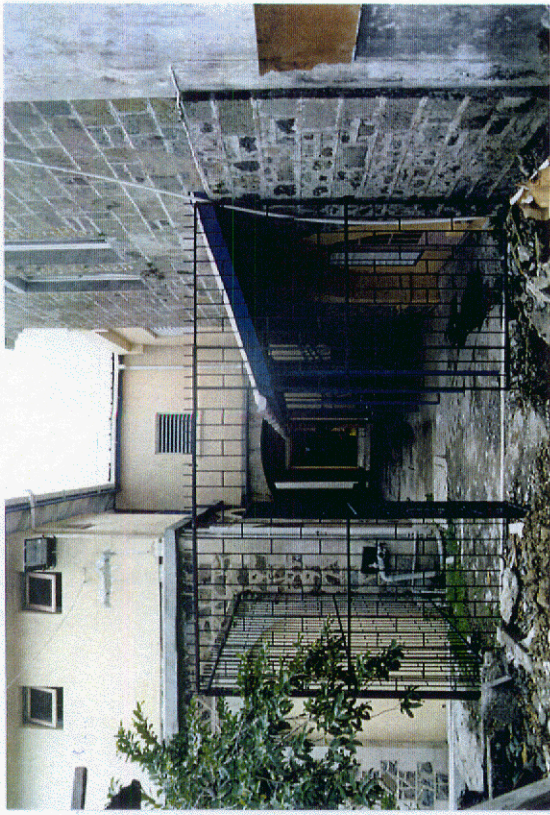
Photo 27: New lean-to shelter roof between Baron Wing and L-Block. The bridge connecting the two buildings is in the background.
