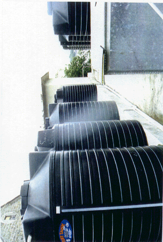
Photo 26: Additional free-standing storage tanks atop roof of existing concrete water tank. They are not fixed to the concrete.
