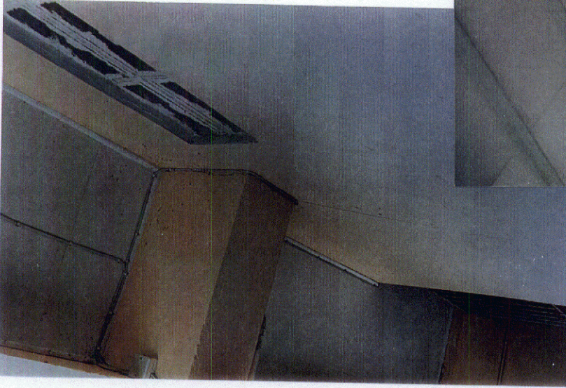
Photo 19: Diagonal crack in infill wall at corner of beam soffit.
