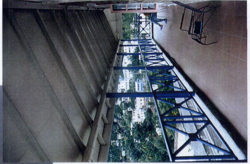
Photo 20: View of verandah of Baron Wing. The new railing is in structural steel, bolted to the concrete upstand.
