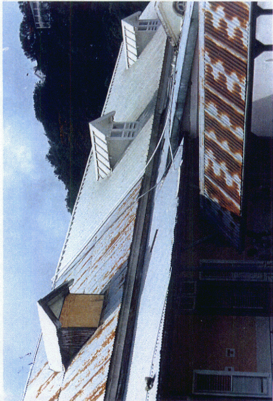
Photo 14: View of renovated and to-be-renovated sections of the L-Block. Cyclone washers have been used on the newer sheeting. Note roof of the "link" in the foreground.
