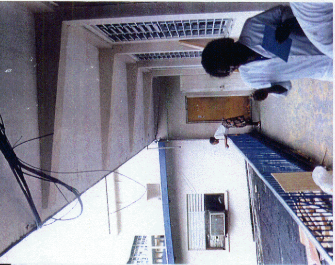
Photo 6: Spalling along the edge of the concrete slab on the Administration Building.
