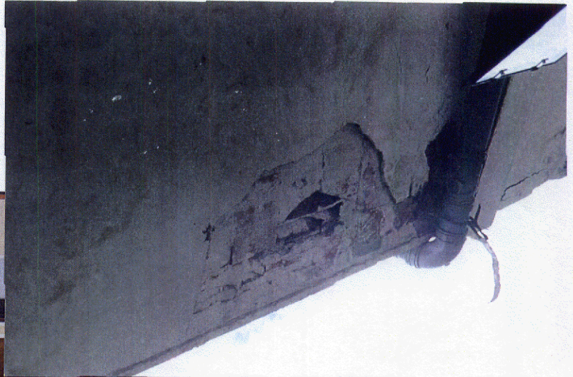
Photo 2: "Drop-out" at soffit of SB slab overhang outside building. Similar instances have occurred inside the building.
