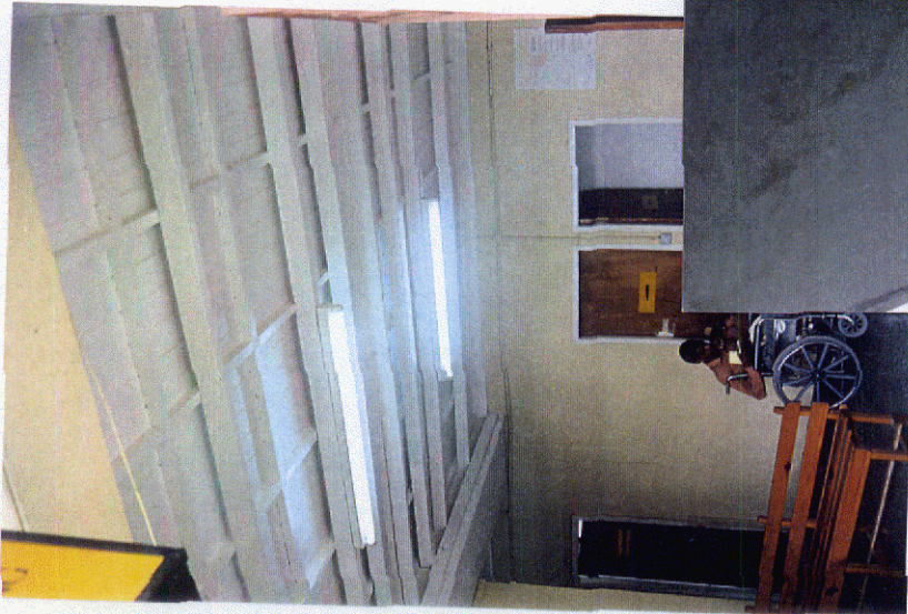
Photo 1: There was a partial collapse of the SB roof in this area. A timber ceiling has been erected here and on other floors to protect occupants from injury in any future collapse.
