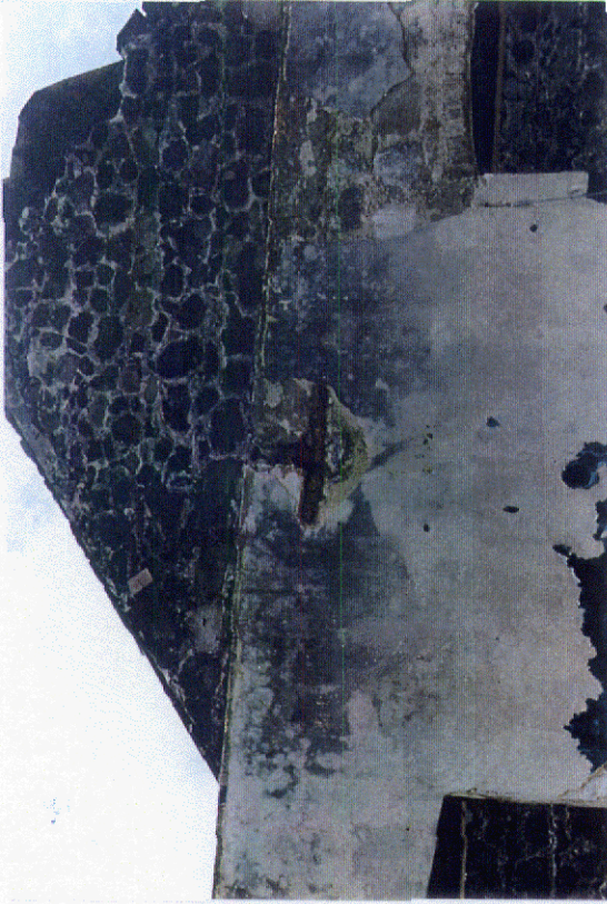
Photo 3: Typical hold-down arrangement at existing truss members on L-Block. There appears to be no connection between the timber and the underlying wall.
