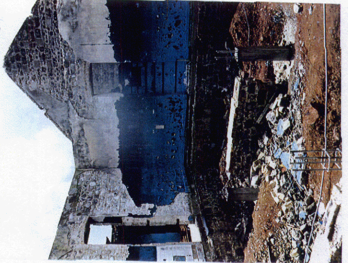
Photo 4: View inside burnt-out section of L-Block. Rubble walls are 16" to 18" thick.
