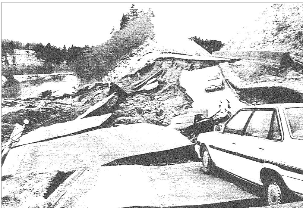
January 16, 1993. Automobiles left on the collapsed national highway after the Kushiro-Oki earthquake. (Photograph provided by Mainichi Shinbun)
