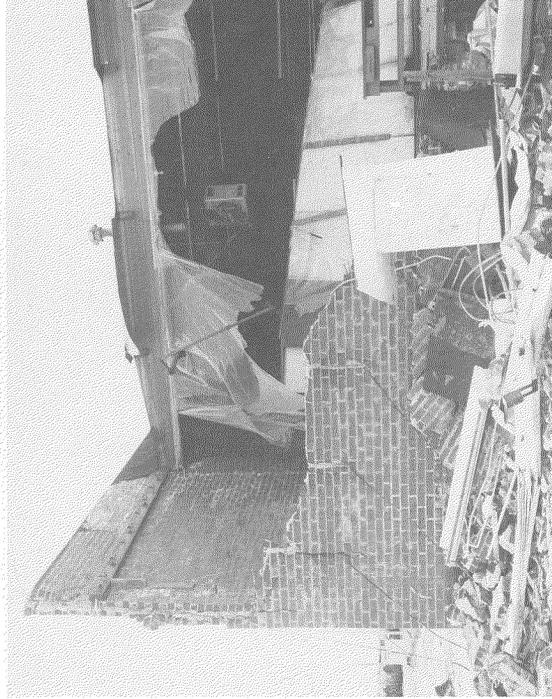
Figure I-8: Typical Industrial Building Damage in City of Sylmar. Average damage to this type of construction in the heavily shaken area was about 17 percent of value. (Los Angeles City Department of Building and Safety photo)
