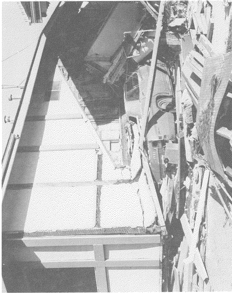
Figure I-9: Collapsed, Split-Level, Single-Family, Wood-Frame Dwelling near Olive View Hospital. Average losses to single-family, wood-frame dwellings in the heavily shaken area were about 7 percent. (Los Angeles City Department of Building and Safety photo)
