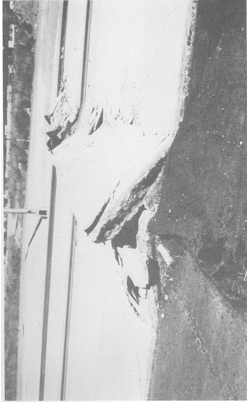
Figure I-6: Buckling of Freeway Pavement Due to Ground Surface Displacements. (C.M. Duke photo)
