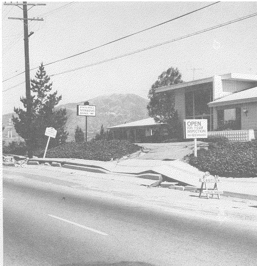
Figure I-5: Surface Fault Break. Area beyond curb was raised about 3 feet relative to the street. Unoccupied nursing home was damaged but did not collapse. (Los Angeles City Department of Building and Safety photo)
