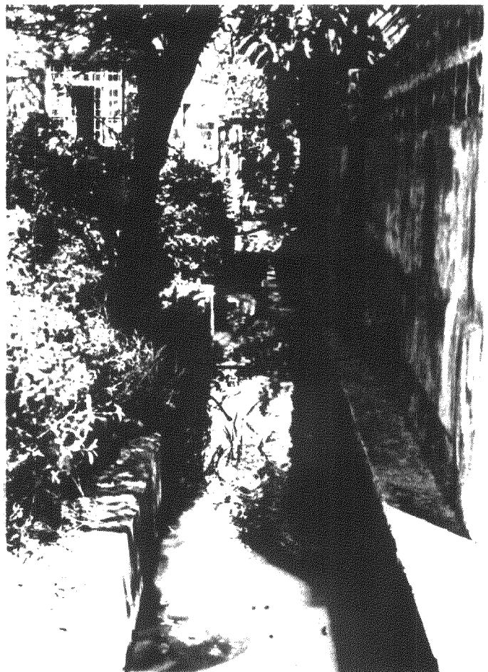
Blocked drainage, close to Victoria street.
